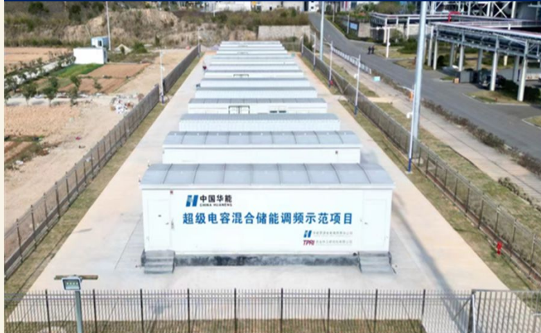
Top view of the demonstration project for frequency modulation of the supercapacitor hybrid energy storage system of the Huaneng Luoyuan power plant
